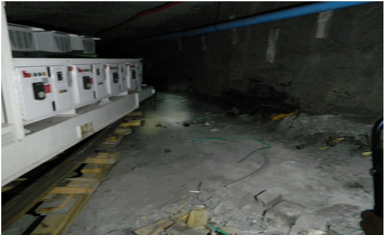
Photos of the Longwall 3MVA Power Car and the accident scene located at 10 Left 16 Block Mule Train Spur
