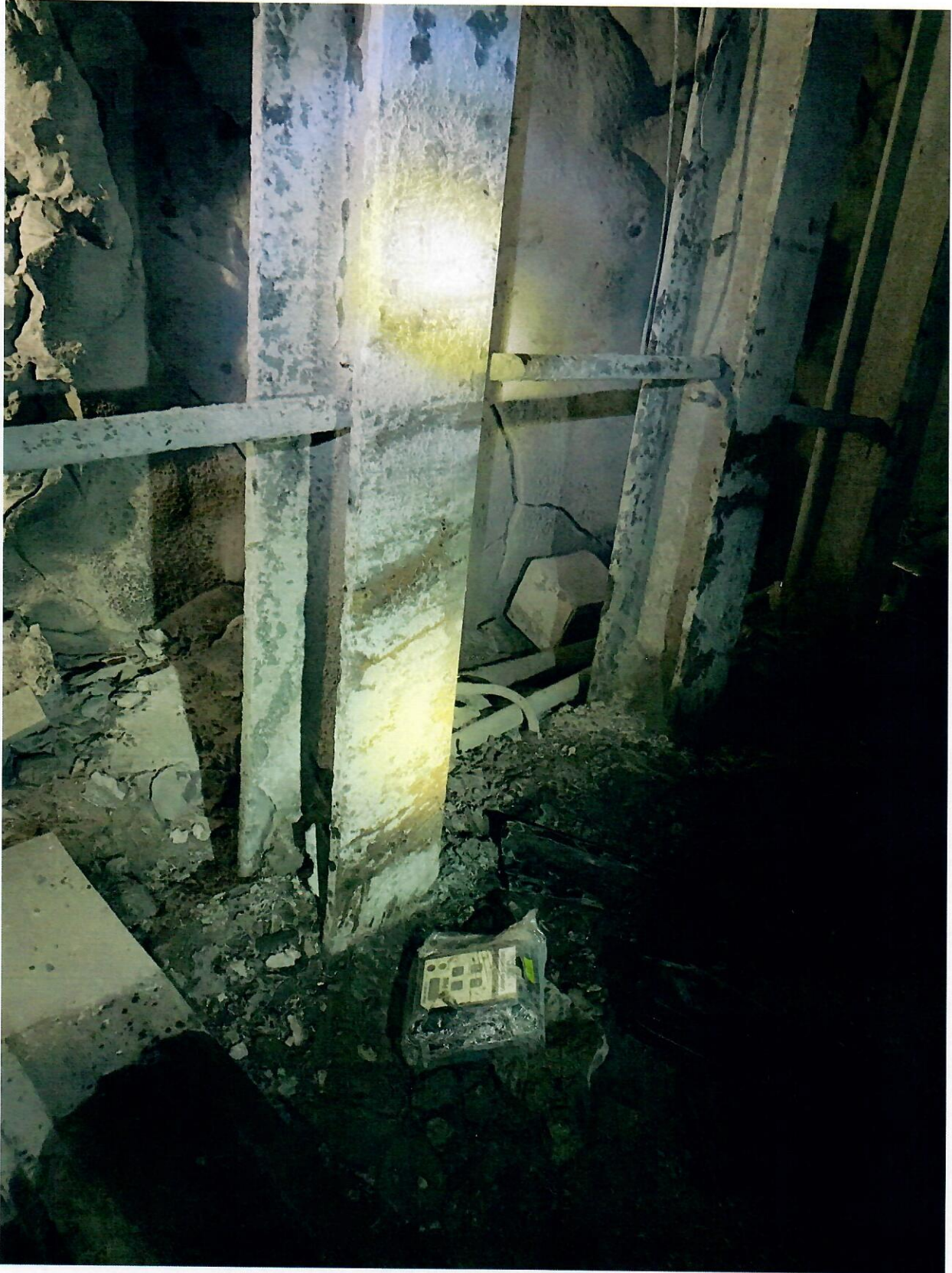
Steel beams at the bottom of slope that the No. 7 EMU collided with during the accident.
