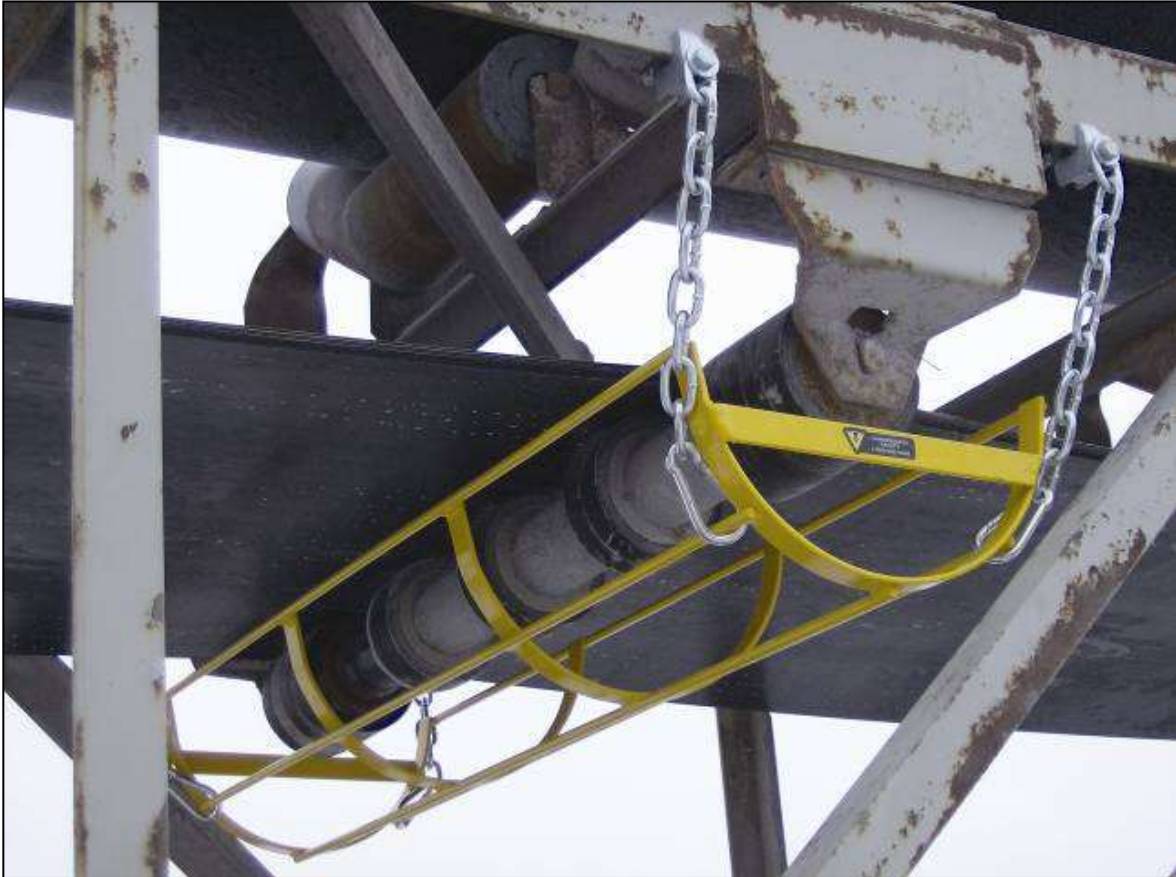
Return Rollers – above 8 feet from the ground.
