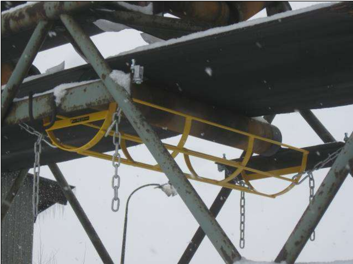
Return Rollers – above 7 feet from the ground.
