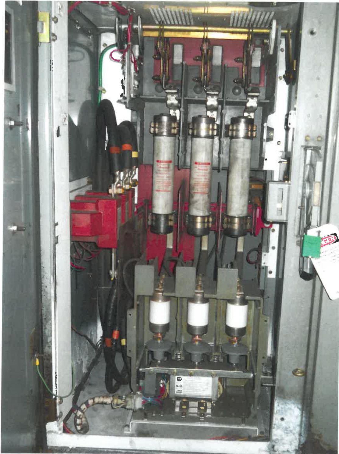
Photo 1.2 Inside of the slope belt A drive cabinet
