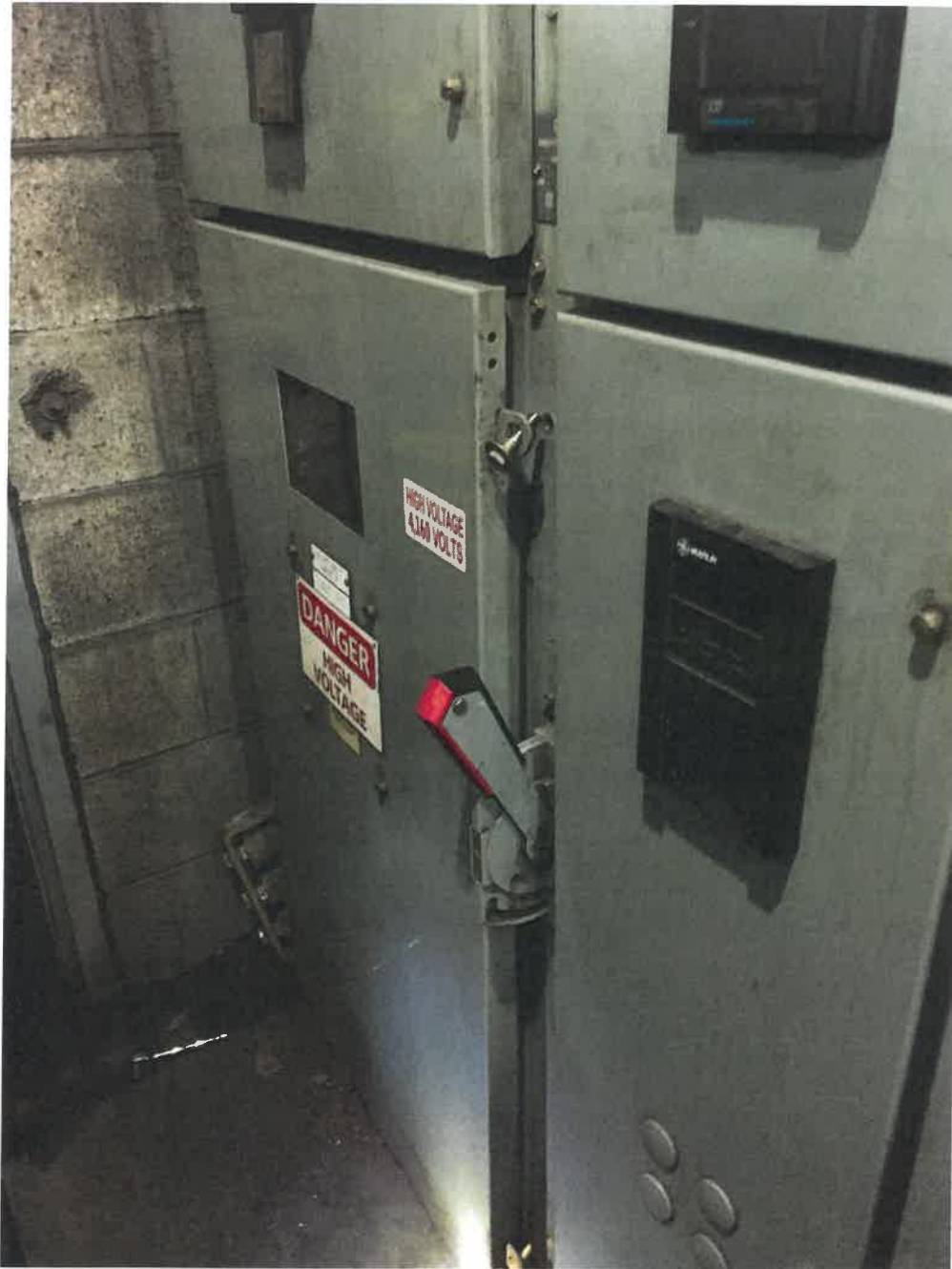
Photo 1.1 Outside of slope belt A drive cabinet
